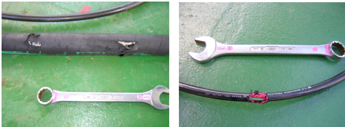
Fig. Q. Ruptured protective sheath (left) and chafed firing line (right).
