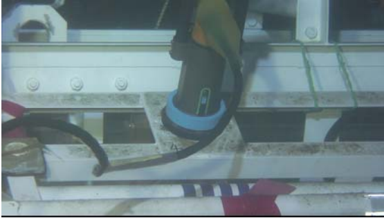
Fig.3-4-3-4 Photo of the junction unit - 2 A galvanic anode and an underwater mateable connector for acoustic reference station
