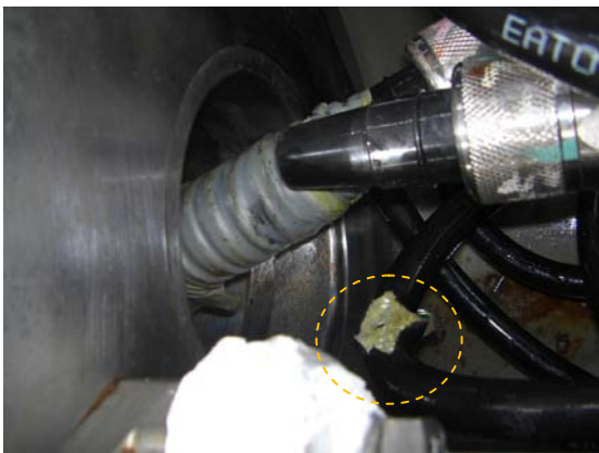
Fig. 4: Damaged air hose rubbed by connector
