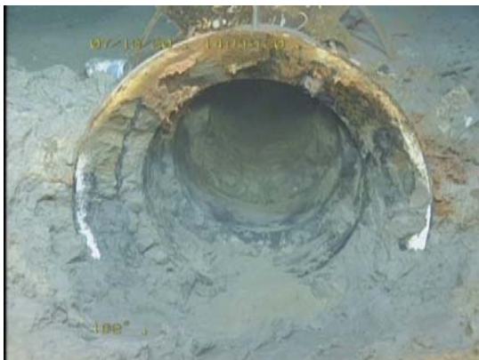
2007(KR07-18) after removing the mud
