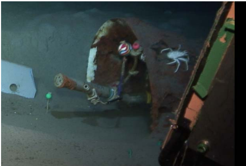
Hydraulic port at the mouth of ACORK head at 808I before connecting the hydraulic connector of the new pressure data logger. Valve is still closed.
