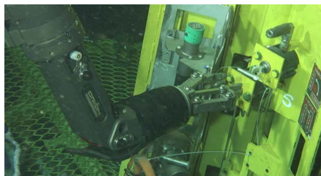
Fig.2-4 the valve was turned to “OPEN”
