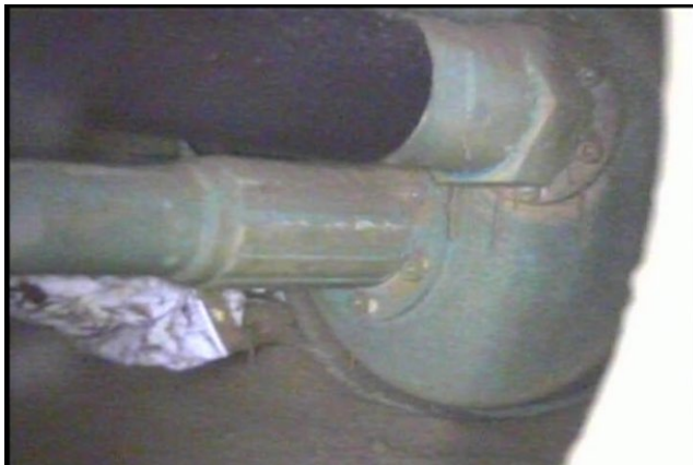
Photo 3.1-3 High-voltage bulkhead connector
