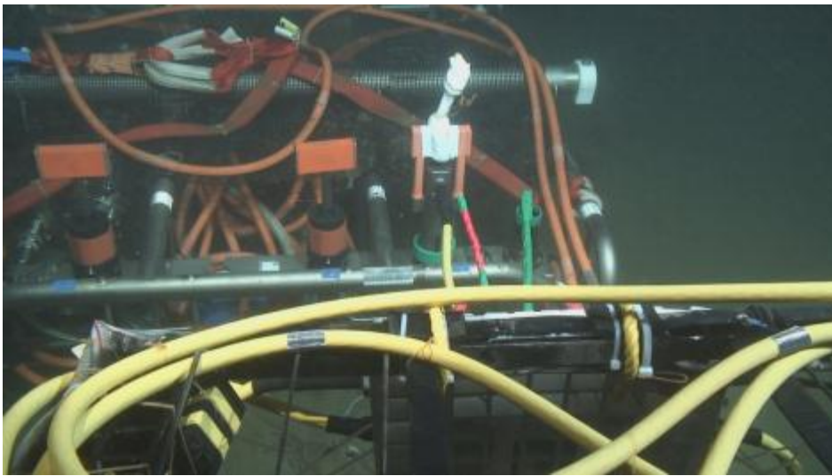
Photo 5 Extension cable interface connecting No.8 port
