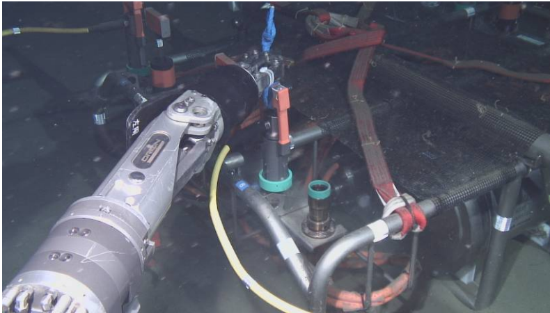
Fig. 3.7 Extension cable interface connecting node B No.8 port
