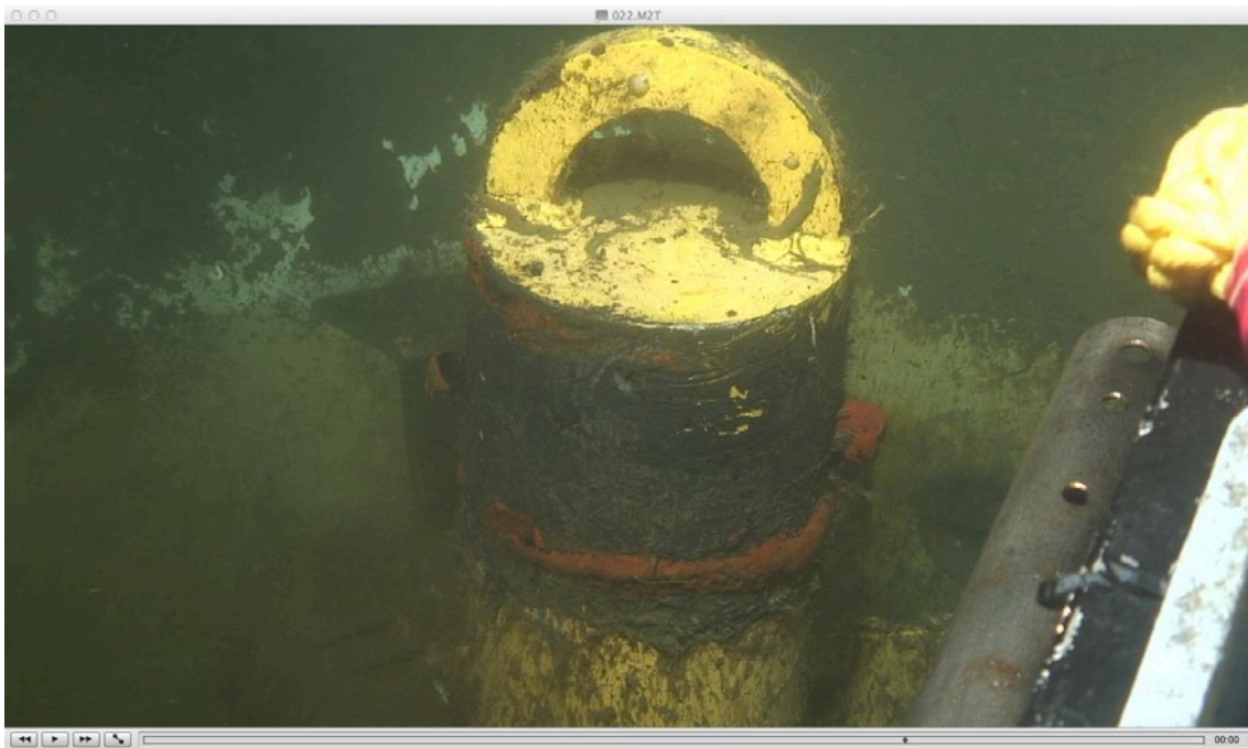
Figure 13. Close-up of the corrosion cap after sweeping with a broom. The part from which the coating was removed by the running tool during installation is only suffered by red rust.
