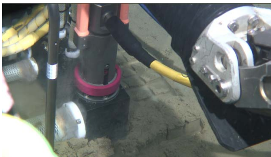
(c) The pressure sensor package and battery were connected.
