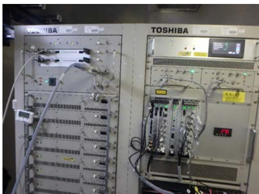
Processing unit of Doppler RADAR.
