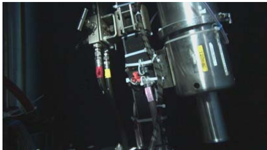
Photo 13 Outlet Flow Meter
