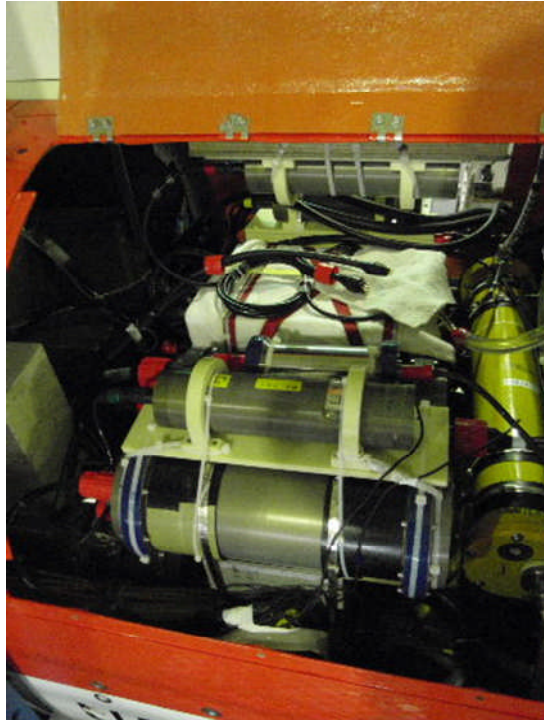
Fig. 5.1.3. Photograph of the payload (from starboard side of AUV Urashima). TX, RX and battery packs were arranged in the payload.
