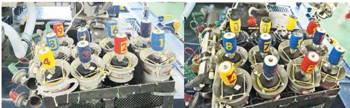
Fig. 3. Two types of the core arrangement viewed from the front bay of 6K.
