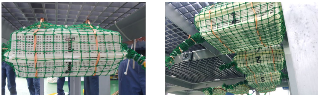
Fig. 6 White basket fixed below the ceiling of the 1 st floor in the platform
