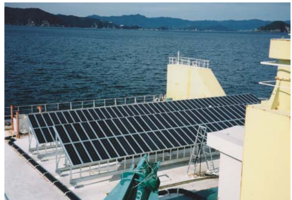
Photo 3 10kw photovoltaic power generation system
