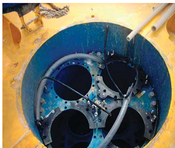
Fig.25 Damage of the Unit No.18 located on the Indian Ocean.
