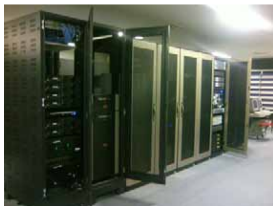
Photo 1 Construction of the infrastructure system for the Biological Information System for Marine Life (BISMaL).
