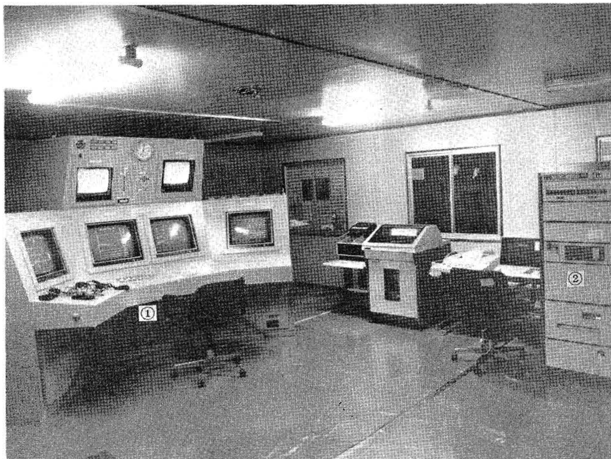
1. 管制卓, instructor console, 2. 計算制御部, computer system
