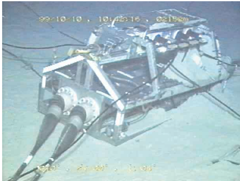
Fig. 8 OBTS after connecting the extension cables. Two cables at near-view are main submarine cables, one to Guam and the other to Okinawa. Top of the frame is the JBX.
